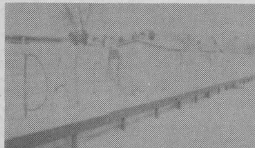
...Graffiti on block walls...
