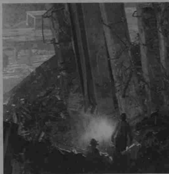
Cutting through the ruins Iron workers use a torch to cut through the twisted steel beams as they continue their search through debris at the site of the World Trade Centre.
