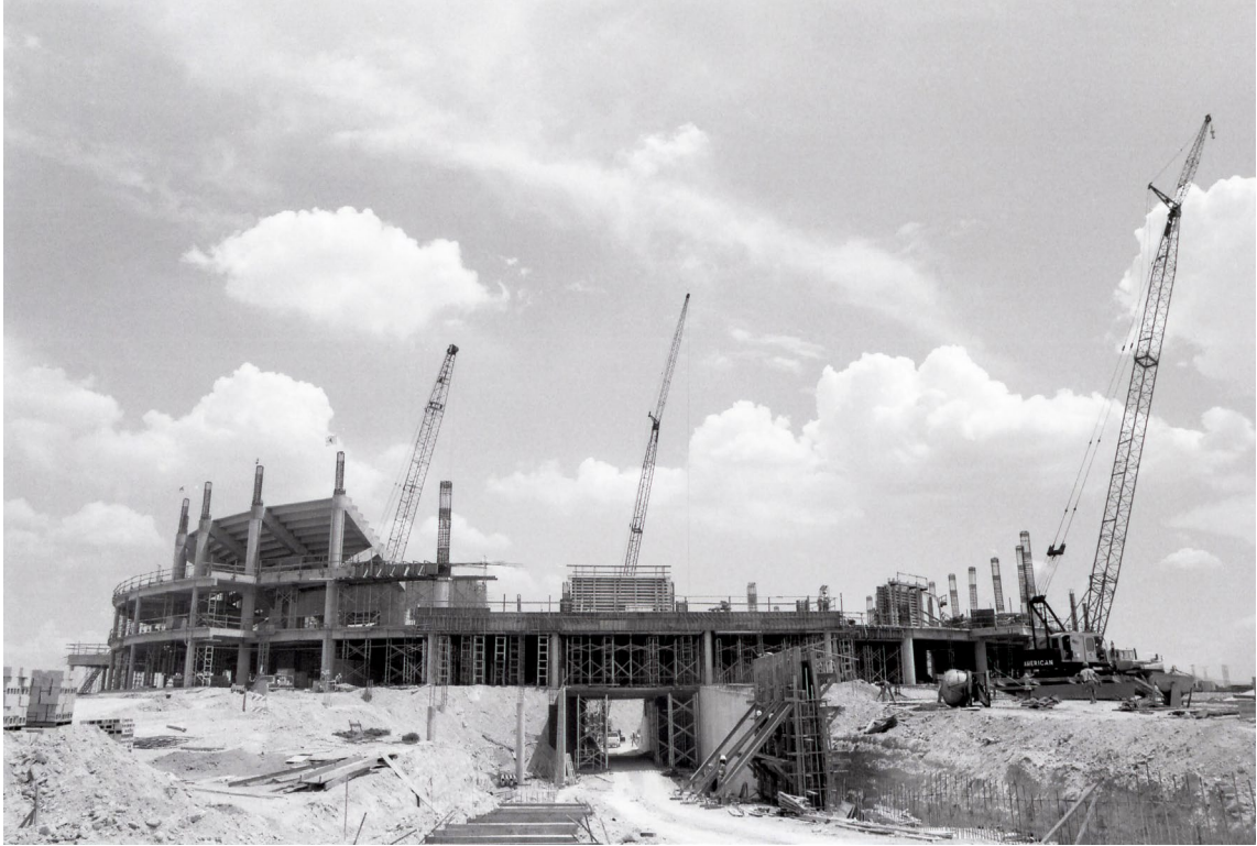
Thomas & Mack construction, July 26, 1982. PH-00388_4782_001.JPG, UNLV Libraries Special Collections and Archives, University Libraries, University of Nevada, Las Vegas.
