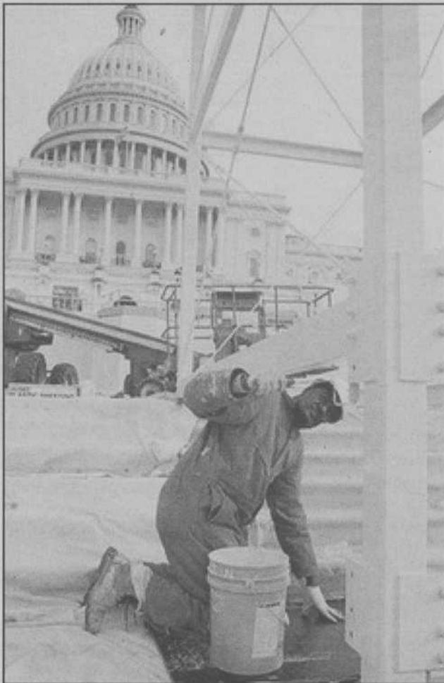
A worker applies a coat of primer on a stand at the construction site of the inaugural stand on the west side of the Capitol in Washington, D.C. The inauguration is Jan. 20.
