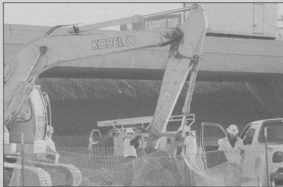
Construction workers continue with a controversial state-approved plan to close "F" Street.
