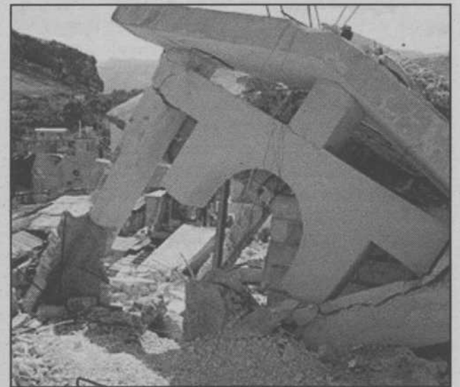
A grade school in central Port-au-Prince partially collapsed Wednesday leaving seven people hurt, Haitian police said.
