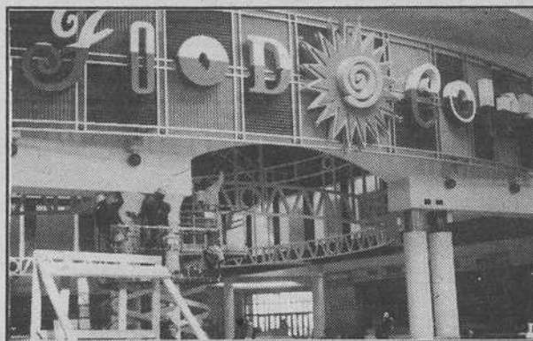
Workers recently apply finishing touches in the new Galleria's Food Court to open next week. Photo by Savoy/LVS-Voice
