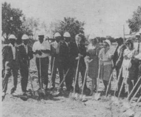
The West Las Vegas Library broke ground on it's new auditorium in August.
