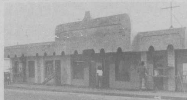
The new exterior renovations of the SURVIVOR'S PLAZA in 1300 block of "D" Street nears completion for tenants (left to right) Andy's Liquors, Religious Emporium, Wesley's Barber Shop and Survivor's Fish.
