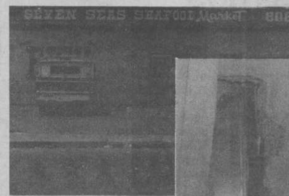
Site Of Burglary Made Over The Weekend At The Seven Seas Seafood (above) And The Created Hole In The Wall (right).
