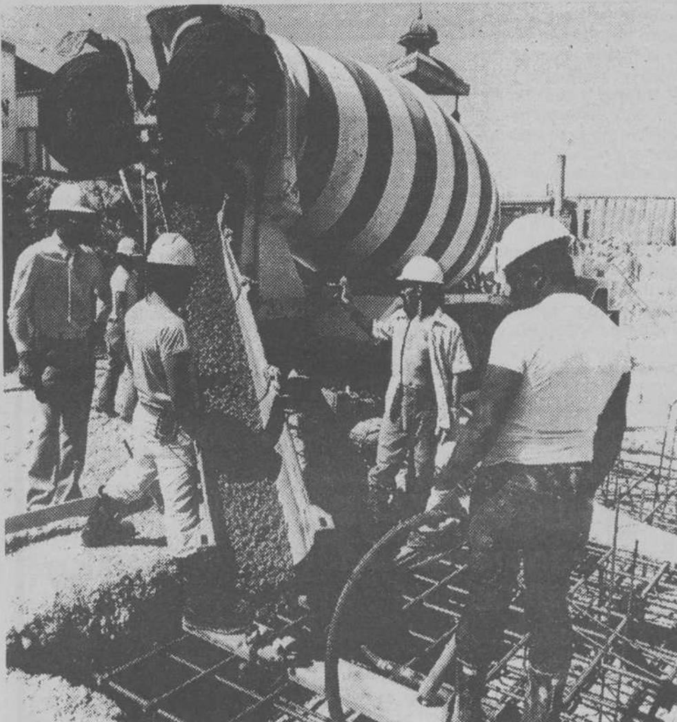
PROGRESS — Jim Roberts, left, project manager of First Western Savings new headquarters, watches workers pour concrete footings of the $10 million building at West Sahara Avenue and Rancho Drive. The five-story building is scheduled for completion in October 1981.
