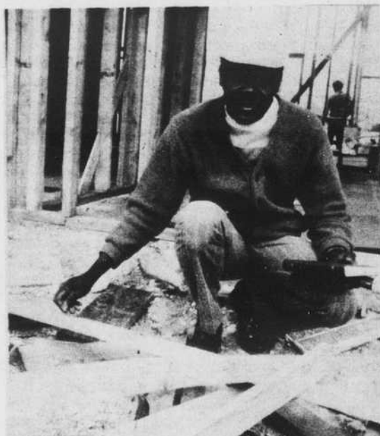
Fred Johnson, NIC Safety Inspector, examines broken section at construction site. Material should have been removed - is tripping hazard.
