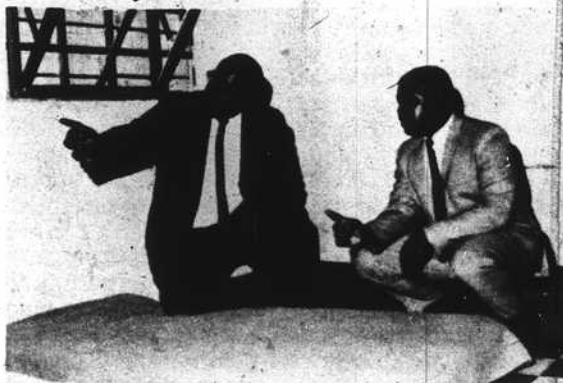
Robert "Moon" Mullen and Don Hampton point out more results of delinquents' destructiveness. Here, windows broken by juvenile inmates, have been replaced with boards.
