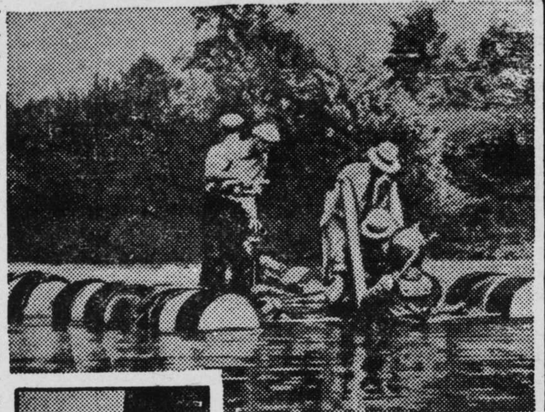
DIVER SUB-MERGING to examine bed of the Juniata River, Pennsylvania, preparatory to laying a pipe line to carry products of the Atlantic Refining Company. Completion of the extension of the system now under construction will link the company's Philadelphia refinery with markets in western New York.
