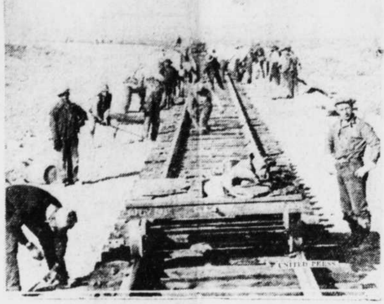
Pictured above is the final stretch of the 23-mile branch railroad between Las Vegas, Nev., and Boulder City. The road, constructed by the Union Pacific at a cost of $1,000,000, connects with the government railroad to Boulder dam. The unit, begun on September 17 with the driving of a silver spike by Secretary of the Interior Wilbur, was thrown open to traffic on February 1.
