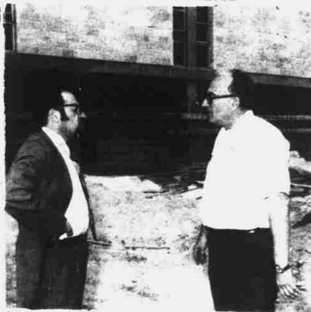
RABBI NORMAN LAMM (LEFT) PRESIDENT OF YESHIVA UNIVERSITY, IS SHOWN THE CONSTRUCTION SITE OF THE NEW SHAARE ZEDEK MEDICAL CENTER IN JERUSALEM BY SHAARE ZEDEK'S DIRECTOR GENERAL, PROF. DAVID M. MAEL. THE OFFICIAL INAUGURATION OF THE NEW MEDICAL CENTER HAS BEEN SCHEDULED FOR THE WEEK OF NOVEMBER 5 - 12, 1978.
