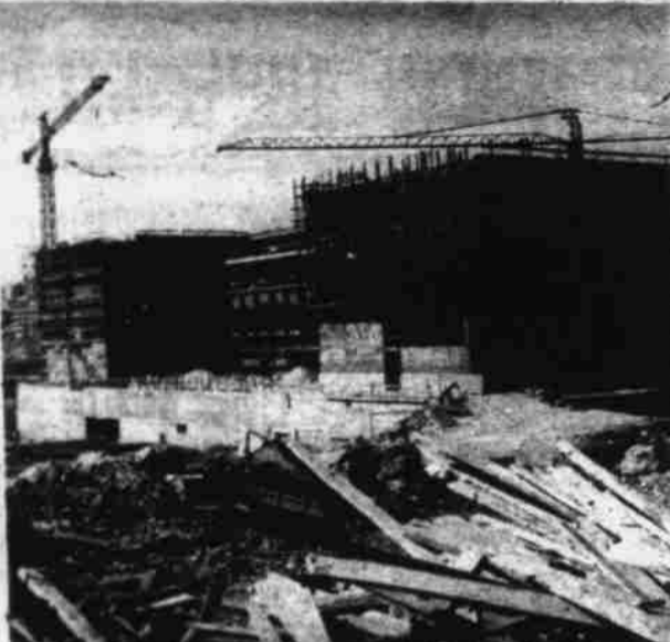
THE NEW SHAARE ZEDEK MEDICAL CENTER IN JERUSALEM RACES UPWARD AS WORK ON THE SKELETON OF THE MAIN AND SOUTHERN SECTIONS NEARS COMPLETION.
