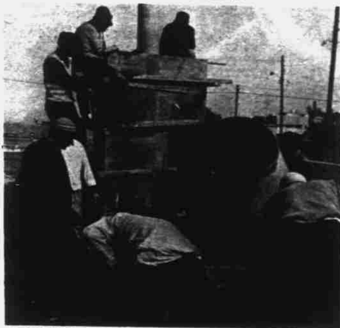
CONCRETE BASES ENCASE ELECTRIC PYLONS FOR PROTECTION AGAINST BOMBS THROWN BY ARAB TERRORISTS IN THE GAZA STRIP. (ISRAEL SUN PHOTO)
