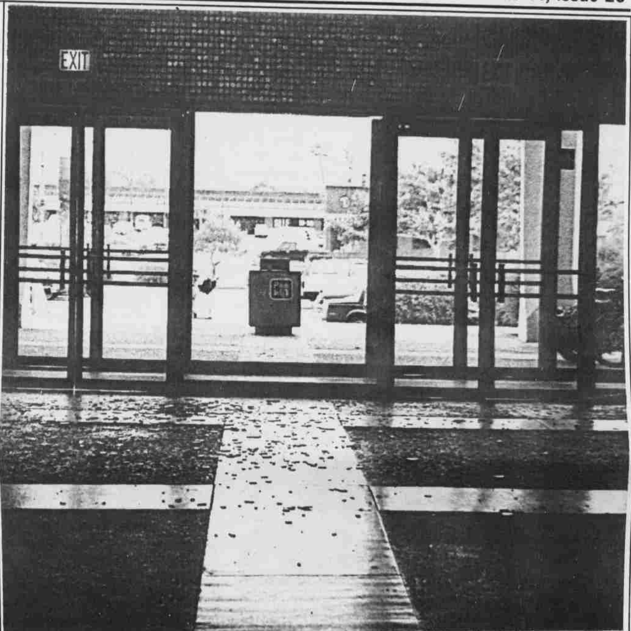
Testimony - UNLV's Flora Dungan Humanities sustained minor damage when the concussion of the blast knocked out a window above the front doors of the building photo by kurt hildebrand, editor
