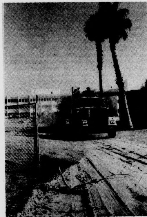
HAUL IT IN — Construction on campus is shown here as a truck is hauling away dirt from the new library edition. It is expected to be open in 1981.
