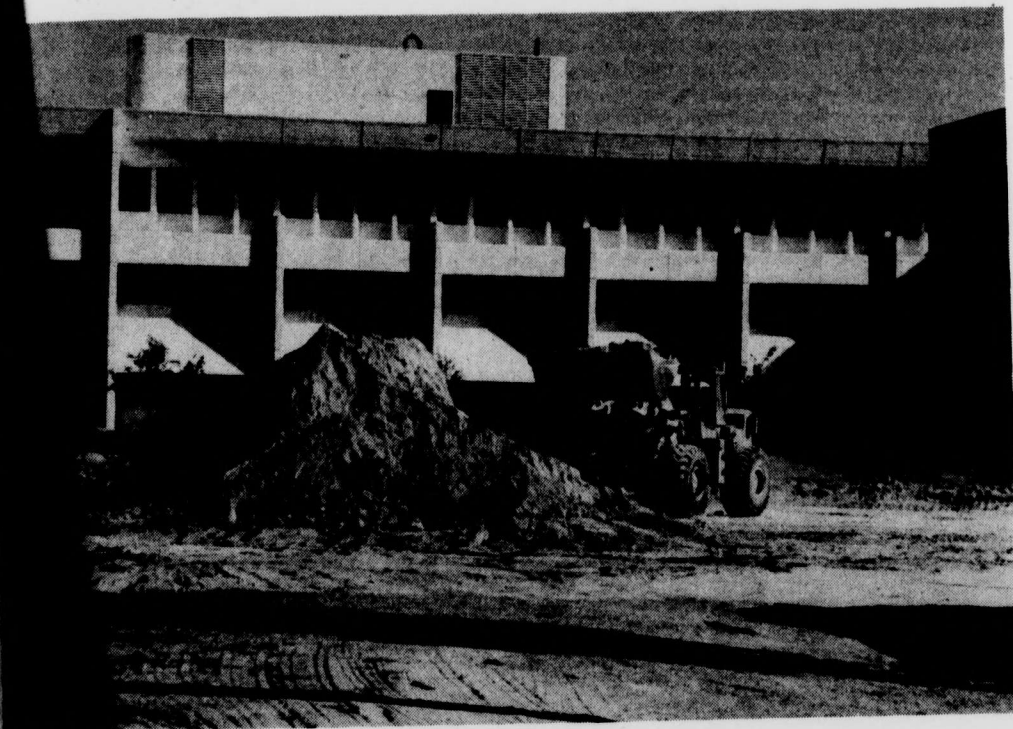
MOVE IT OVER — Construction on campus is almost as bad as on the Strip. Here a tractor is moving dirt
