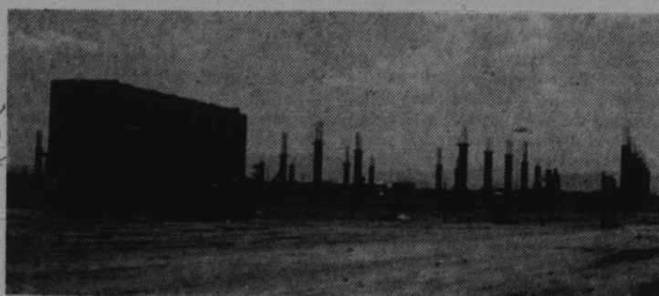
SUB SURFACES AT NSU — Student Union Building, that is! Construction on the Union was begun last month, shortly after graduation. The facilities are scheduled to open for use in June, 1968.
