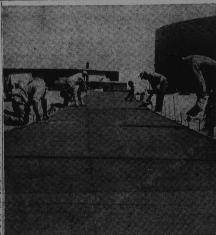
SIDEWALKS GOING IN — Construction workers are putting the final touches on the long awaited sidewalks that are finally being installed connecting the various buildings on campus. (See story below.) (Photo by Mike Gordon)
