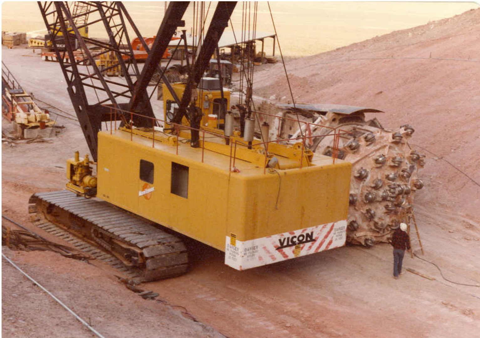
32 – Area 25 at Little Skull Mountain in front of X-Portal with a Tunnel Boring Machine
