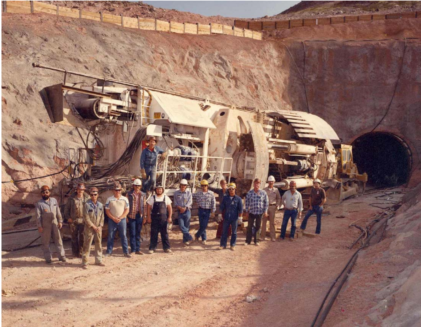
31 – Area 25 at Little Skull Mountain in front of X-Portal with a Tunnel Boring Machine
