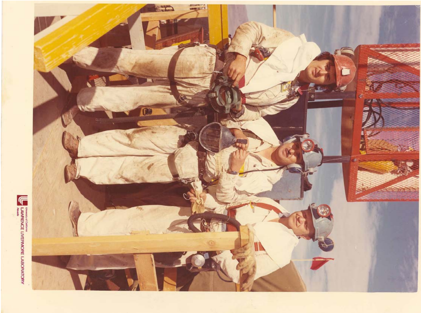
U7AK cased hole – cable repair on the arming and firing cables on test code named Esrom (Right to Left are John F. Campbell, Anselmo Fresquez, and Phil Pinter)
