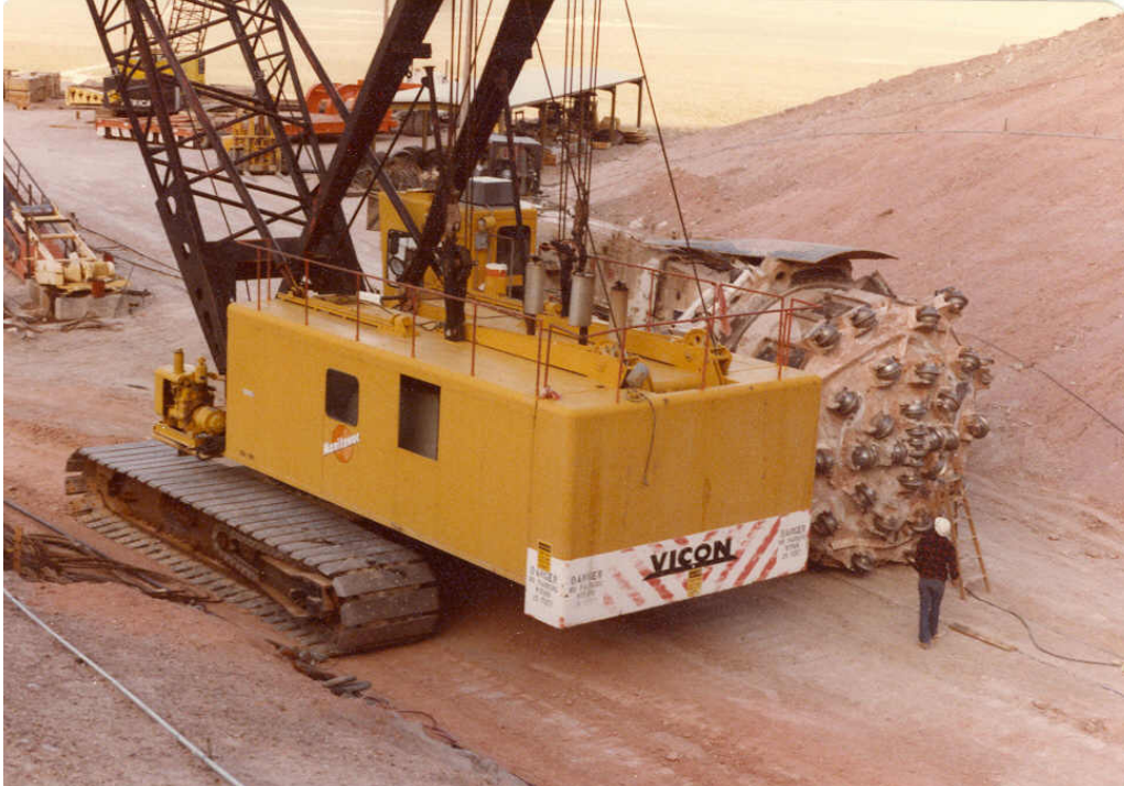
32 – Area 25 at Little Skull Mountain in front of X-Portal with a Tunnel Boring Machine
